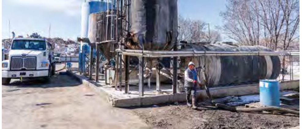
This photo with Jorge Mendoza shows a wider view of the dewatering system from Aqua-Zyme.
